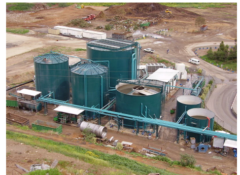
Figure 20.2: An Anerobic digestion plant, Tel-Aviv
