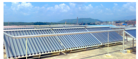
Figure 33.3: Industrial solar water heaters, India
