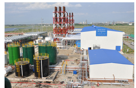
Figure 4.3: An example Liquid Fuel Power Plant
